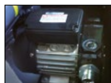
Automatic-manual fuel transfer pump
